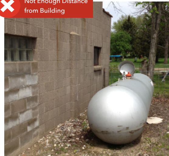
1000 Aboveground Gallon Propane Container
